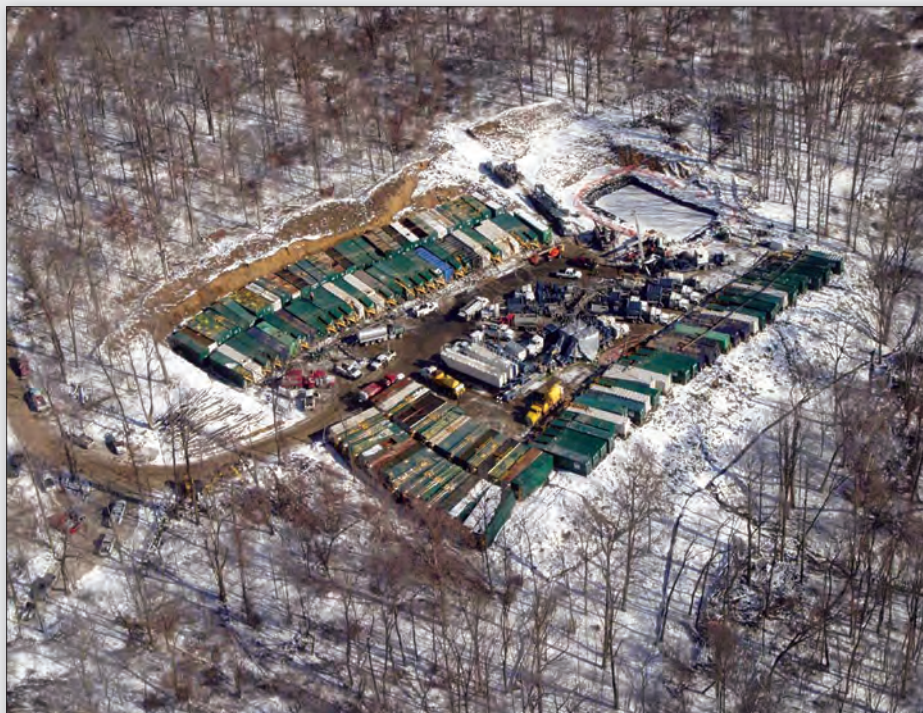
Figure 6. A hydraulic fracturing stimulation in 2007 on a Marcellus Shale gas well showing the amount of equipment involved.
