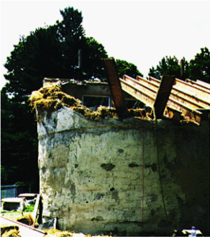
Figure 8: We began removing the I-beams from the side and worked our way toward the middle.
