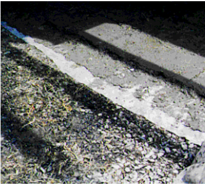
Figure 1: The four layers in the floor: 6 in. of unwashed gravel overlain with 6-mil polyurethane sheet, topped with flagstone slabs potted in about 1/2 in. rock dust
