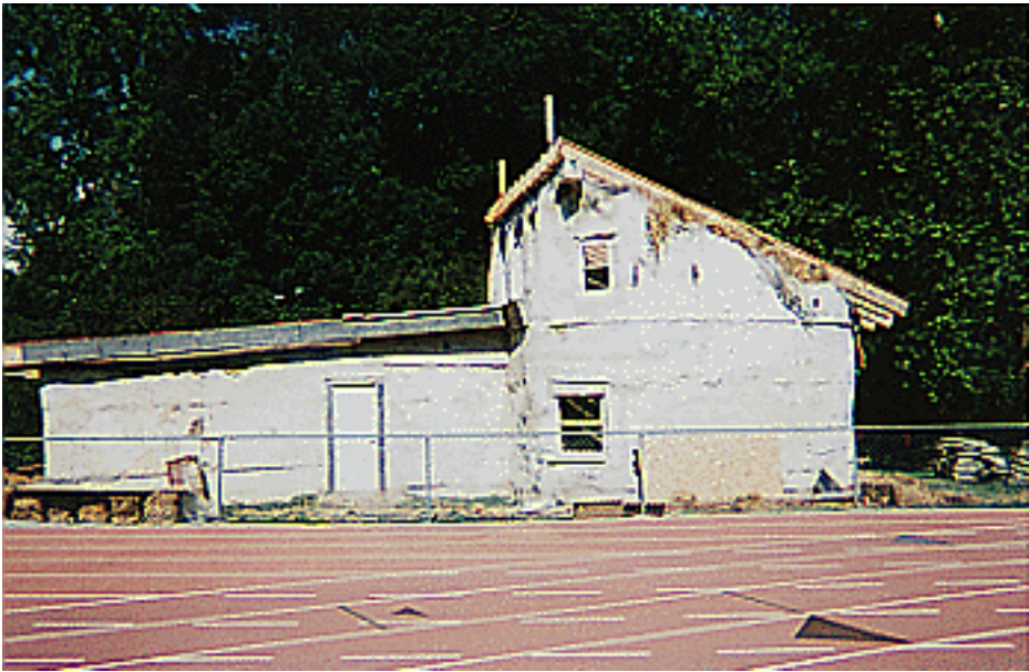
Figure 6: Removing the roof on the circular room was a formidable task because of the steep incline.
