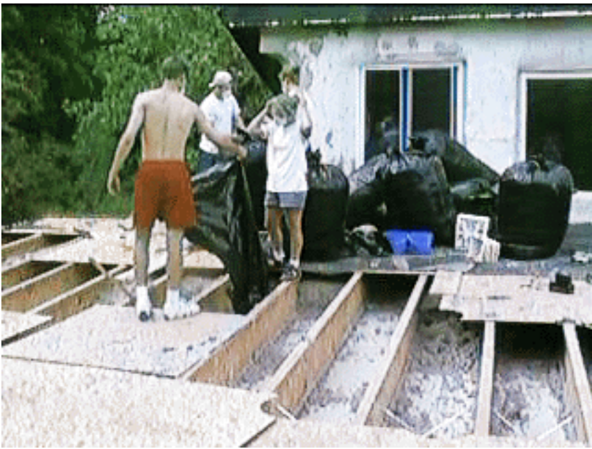
Figure 4: Seen at the bottom of the channels are the sheets of drywall which were too fragile to be taken down in complete pieces.
