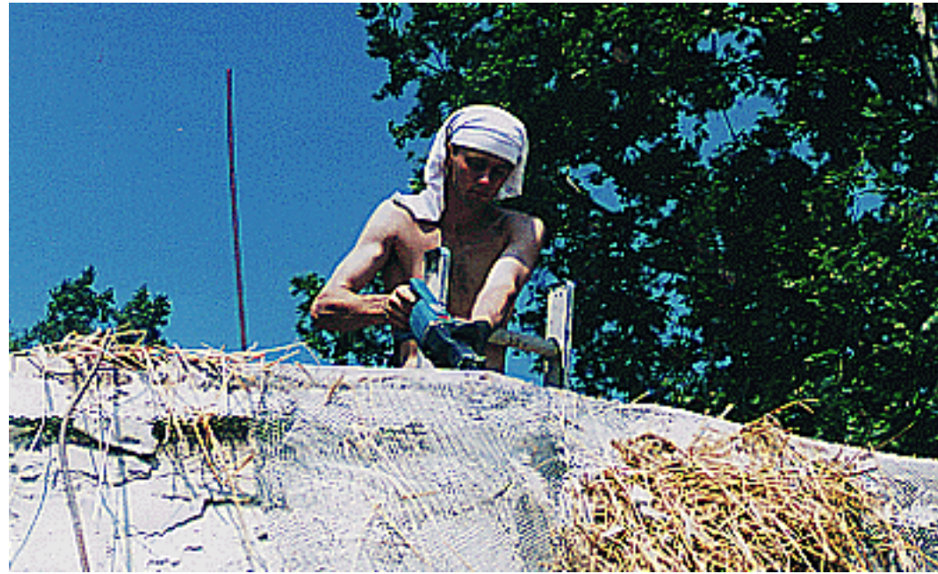
Figure 4: A worker cuts the bond beam into sections. As the bond beam is pushed off the top of the wall, it would pull down the wire lather connected to it.
