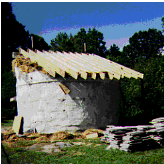
Figure 7: The roof of the circular room after all decking and insulation had been removed.
