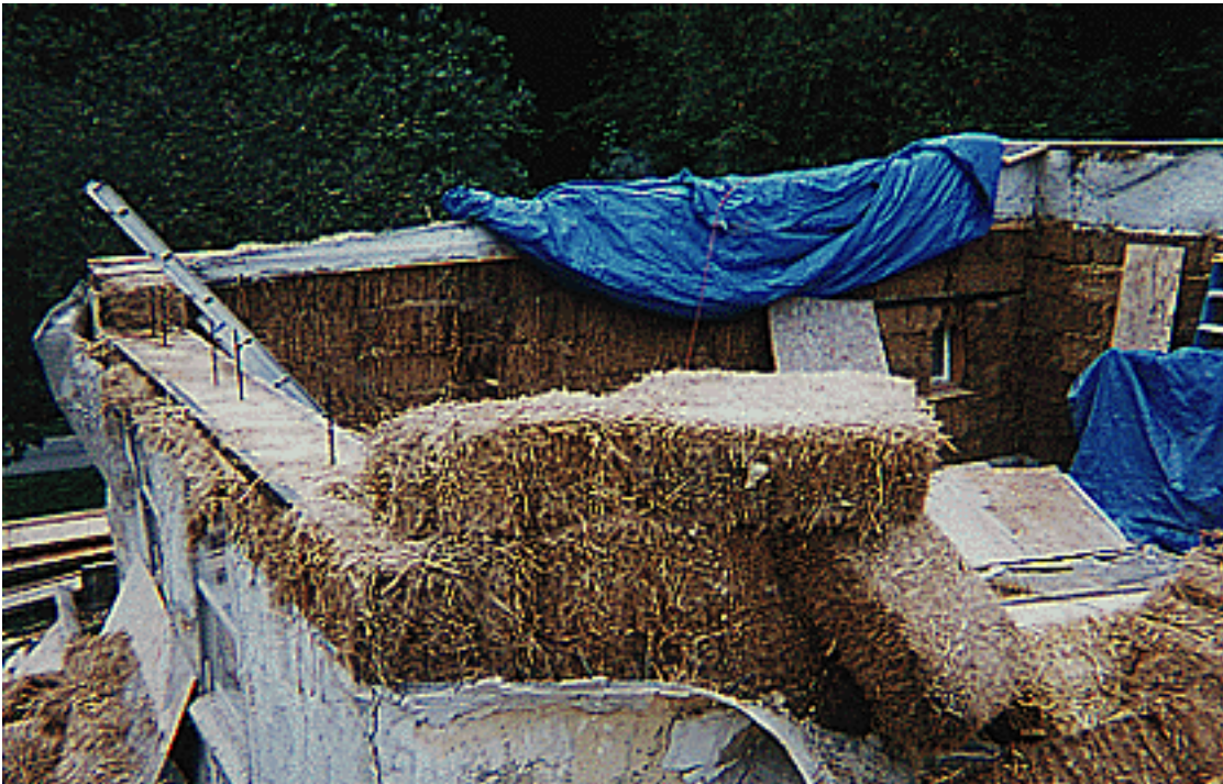
Figure 1: Seen here is the bond beam on top of the rectangle wall.
