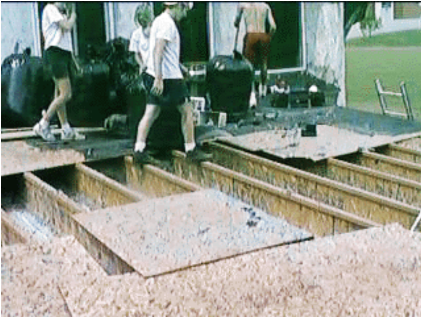
Figure 5: The remaining roof at the top of the picture was left intact to support a ladder which would lead to the top of the roof of the circular room.
