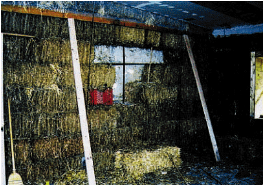
Figure 3, showing four bales removed, with poles (and plastic milk crate) holding up weight of bales above removed ones. Visible in the hole is the underside of the galvanized diamond lathe holding exterior stucco.
