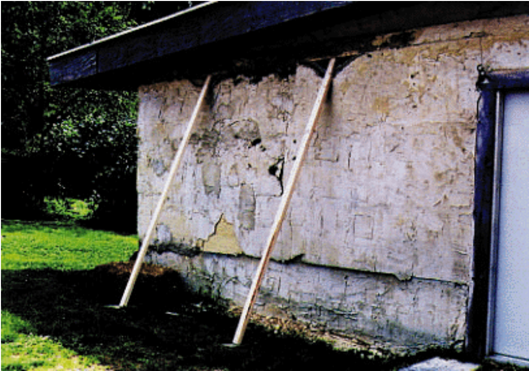
Figure 4, showing outside stuccoed wall after removal of bales. The stucco is cracked and would have to be re-laid after the operation.
