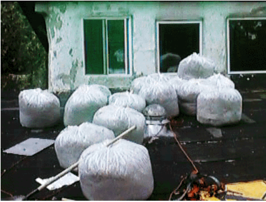
Figure 3: Shown here are bags of blown cellulose insulation ready to be transported for reuse.
