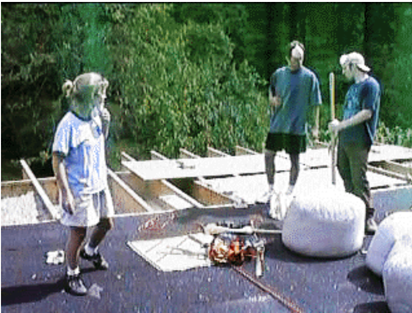
Figure 1: student workers peel off asphalt roll-roofing and pry up oriented-strand-board four-by-eight sheets (1/2 in. thick) to reveal channels holding blown cellulose insulation.
